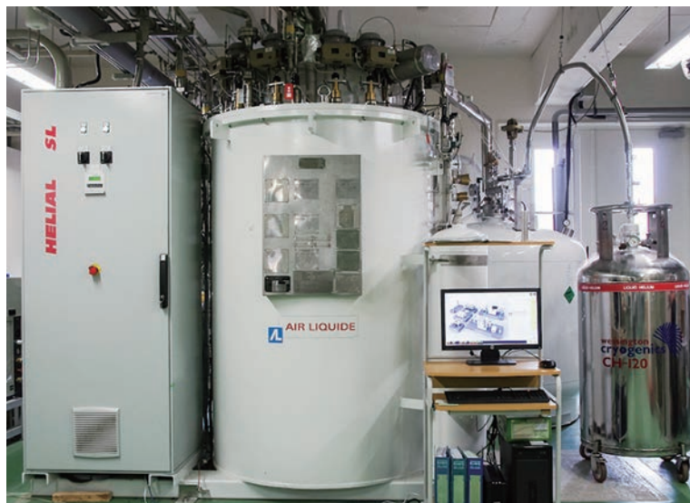
Fig. 1: Helium liquefier in CL
