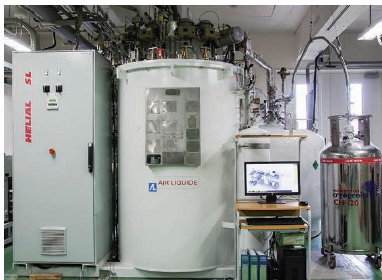
Fig. 1: Helium liquefier in CL
