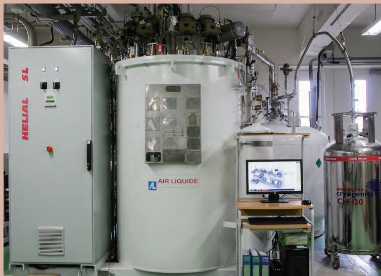
Fig. 1: Helium liquefier in CL
